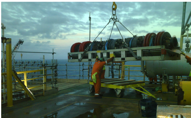
Jee Ltd: Lifting operations for 34 in. TDW SmartPlug prior to loading (operation project managed by Jee).
