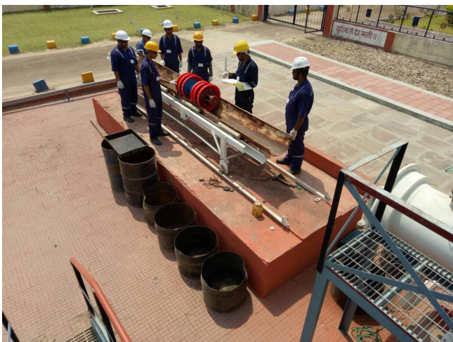
VKVC LLP: VKVC foam pig near the receiver end after successful removal of the stuck pig.
