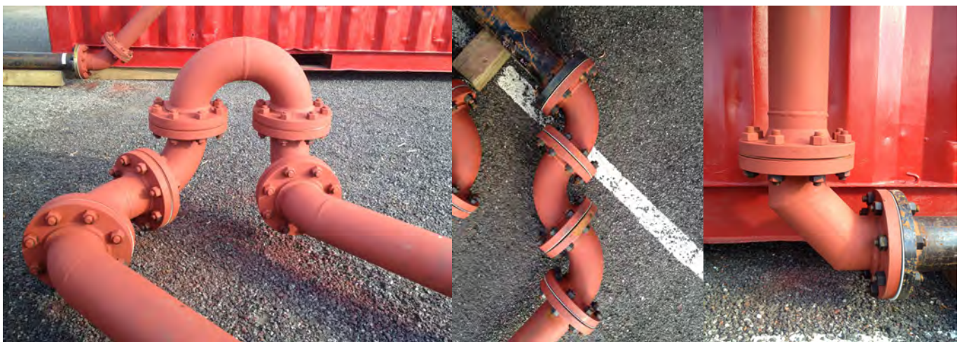
Figure 1. Examples of various complex piping configurations once deemed unpiggable.
