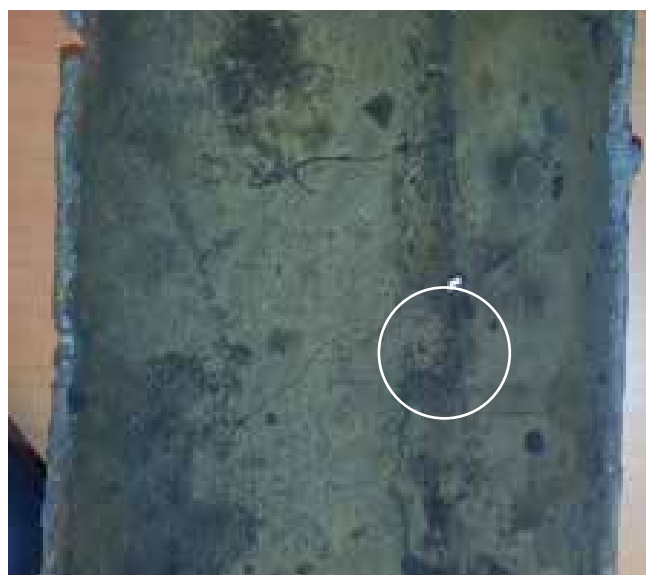
Figure 2b. Two Additional Areas of Internal Localized Wall Loss
