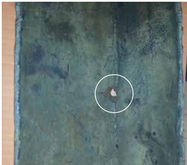
Figure 2a. Hole in Tube Causing Premature Leakage in Piping
