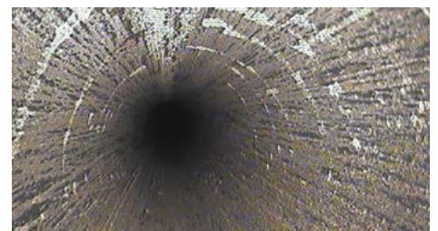
Figure 1. RVI visual images show the extent of the damage within the convection section of the piping.
