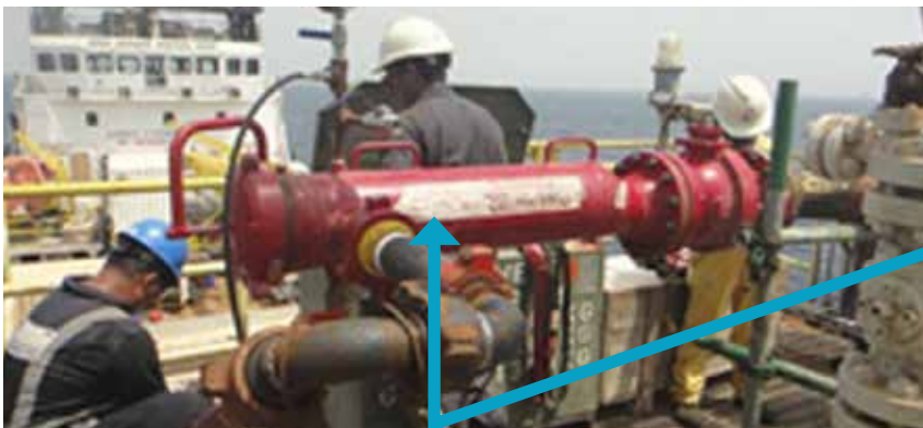
A temporary launcher connected at the blind flange
