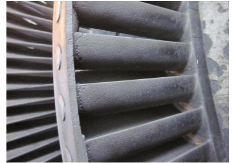
Figure 1. Corrosion damage on geothermal steam turbine blades
