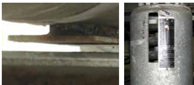
Malfunctioned hangers or supports
