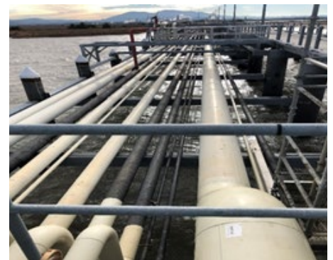
Wharf lines operated by Andeavor Logistics LP at the Avon Oil Terminal, fronting the Suisun Bay near Martinez, Calif.
