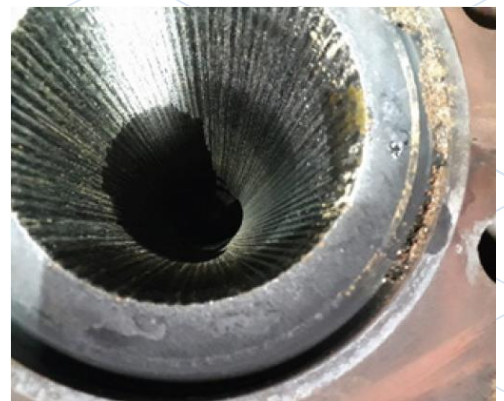
Figure 9. Damage (grooving) on tube internal surface from over-cleaning
